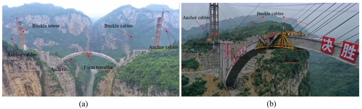
Figure 9. The site construction of Jiming Sansheng Bridge: (a) Panoramic view, (b) Partial view.
