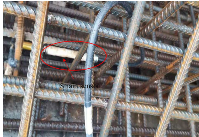
Figure 17. The scene of the concrete stress sensor.
