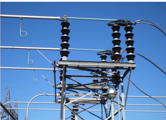
Fig. 9. BPA 230-kV line entrance gaps.
