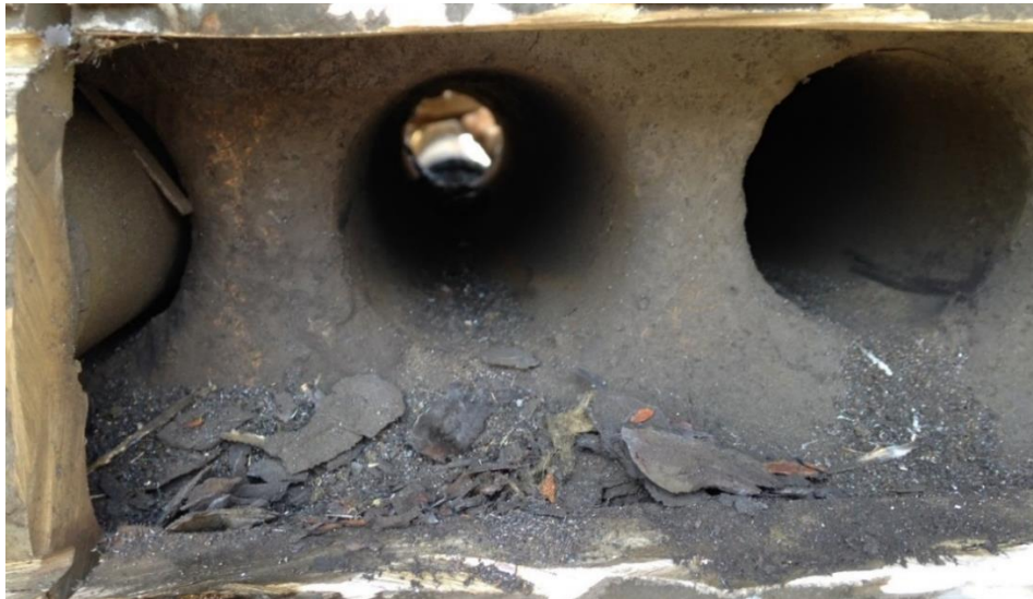
Fig. 2.4: View of the cut tube sheet marked as TS 3 in Fig. 2.2. Position 3 rd row, tube 4 and 5. No abnormality is seen.
