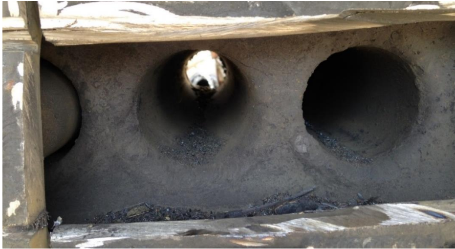
Fig. 2.3: View of the cut tube sheet marked as TS 2 in Fig. 2.2. Position: 2 nd row, tube No. 3 and 4. No abnormality is seen.
