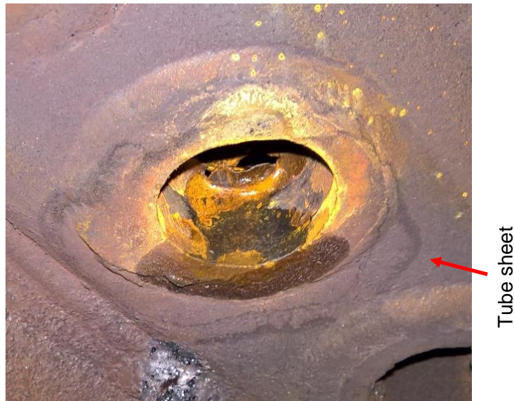
Fig. 1.5: View of the damaged TLE tube of furnace 5, TLE A. Almost the entire circumference of the tube was almost damaged (location is 3-4 cm away from tube-sheet).
